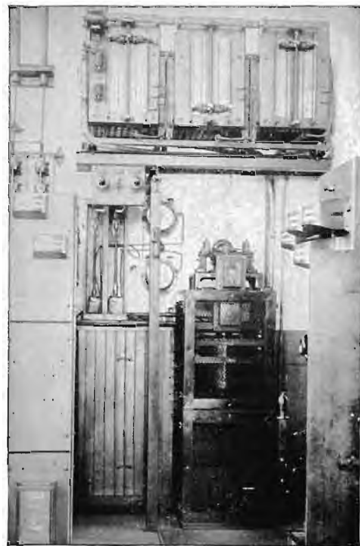
POWER LIMITING AND INDICATING EQUIPMENT INSTALLED IN SUBSTATION
