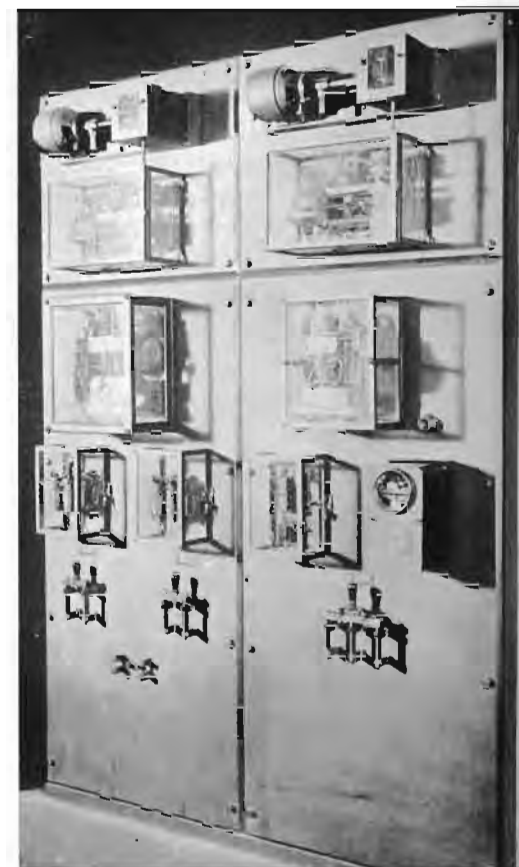
POWER INDICATING AND LIMITING BOARD AT THE DISPATCHER'S STATION, TACOMA
