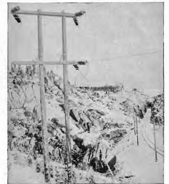
ANGLE TOWER ON 100,000-VOLT TRANSMISSION LINE
