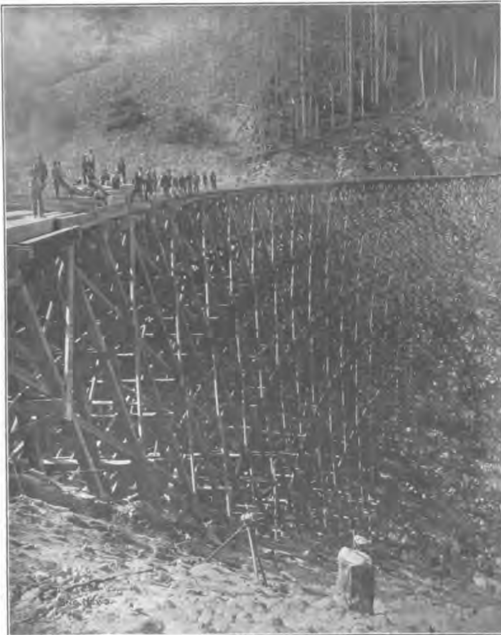
FIG. 2. A TIMBER TRESTLE, 190 FT. HIGH, ON THE PACIFIC COAST EXTENSION OF THE C., M. & ST. P. RY.
