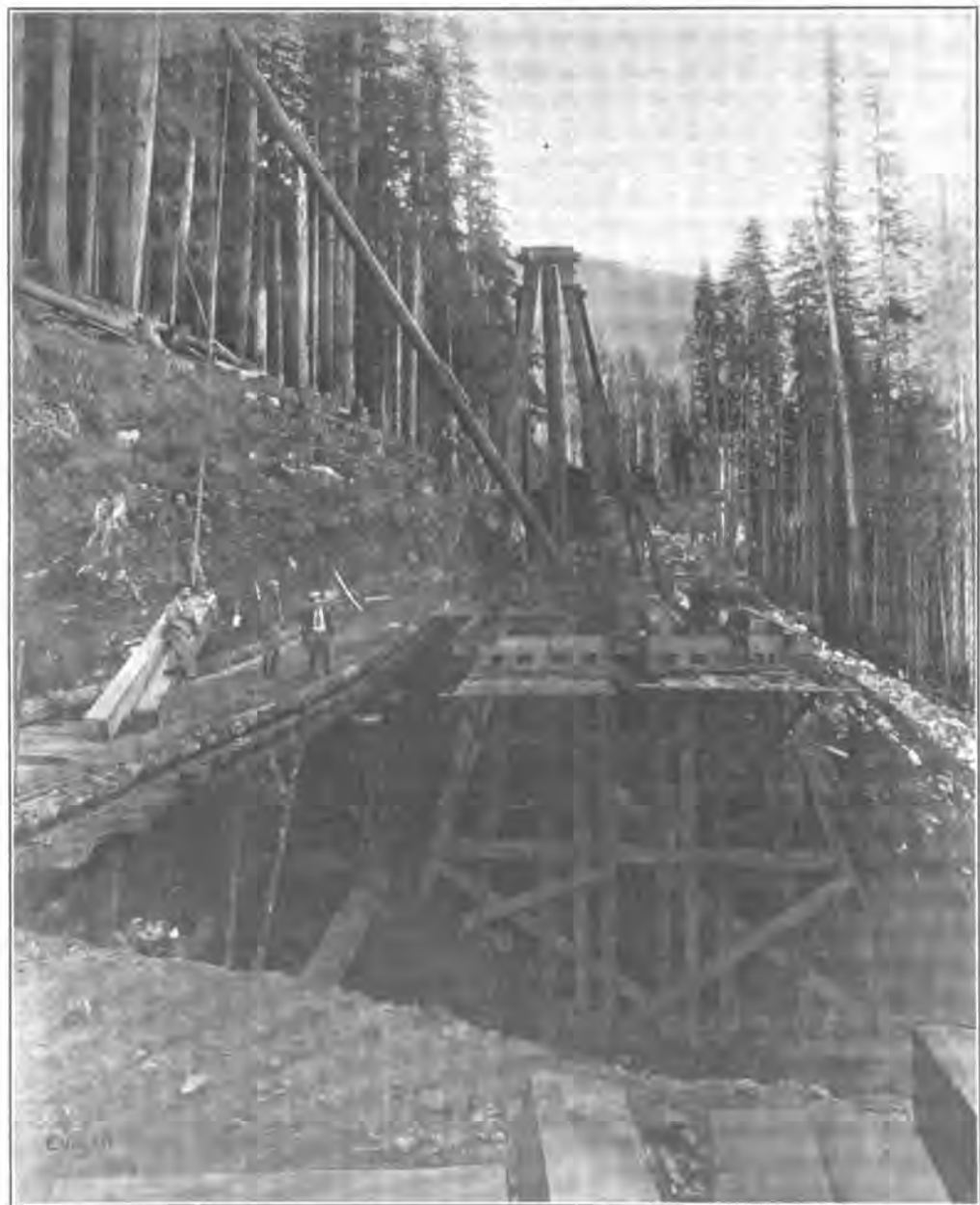
FIG. 4. START OF CONSTRUCTION OF TIMBER TRESTLE ON NEW LINE IN STATE OF WASHINGTON.
