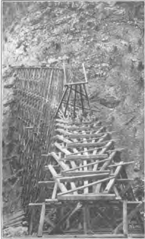
Fig 3. Method of Erecting Timber Trestles on Snoqualmie Line of C., M. & St. P. Ry.
