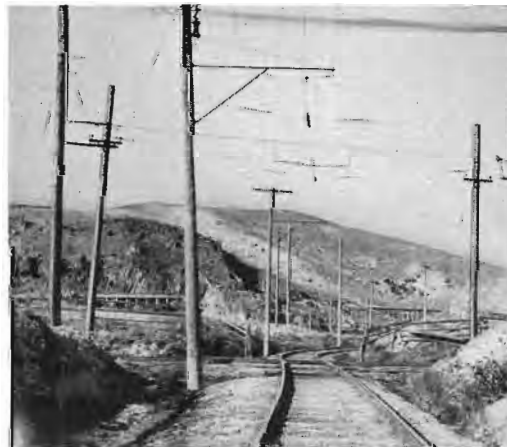
INTERSECTION OF 2400-VOLT SYSTEM WITH TROLLEY CROSSING
