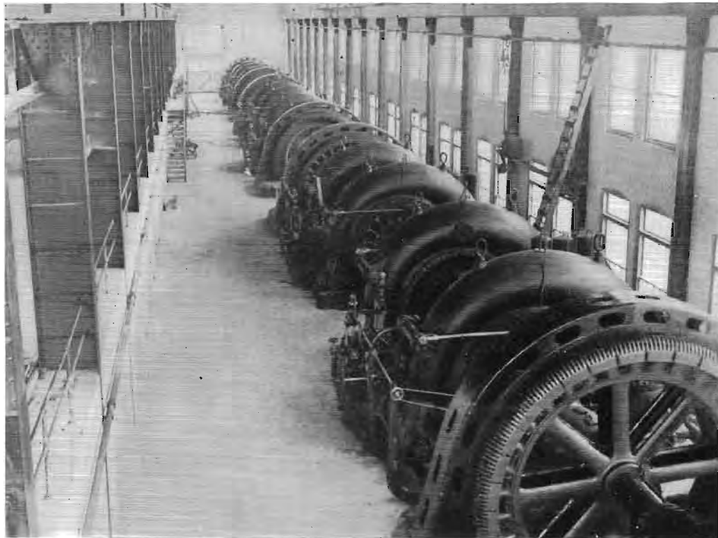
GENERATOR ROOM IN THE RAINBOW STATIONS OF THE GREAT FALLS POWER COMPANY
