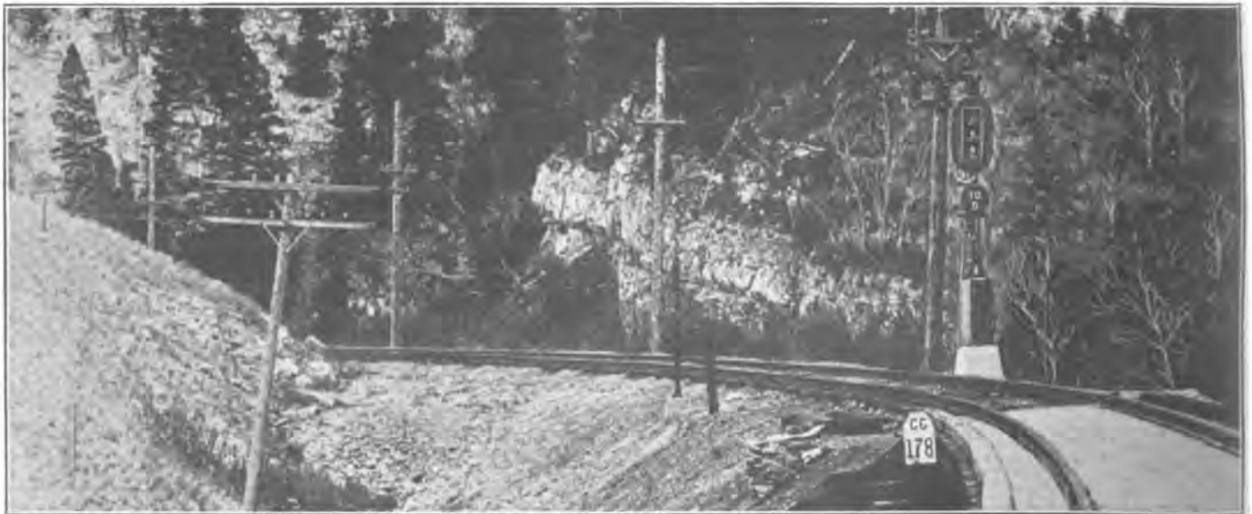
Typical Three-Light Signal With Line Transformer on Pole in Background.
