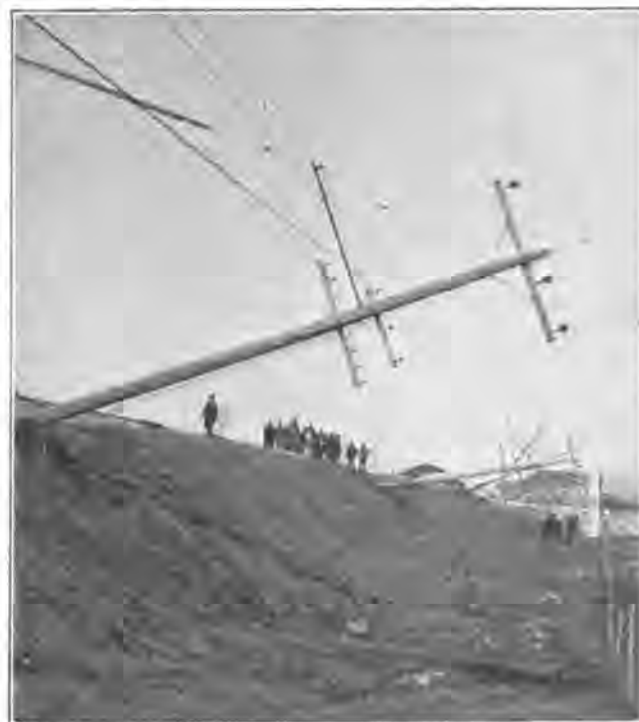
HIGH-TENSION POLES BLOWN DOWN ON THE KANSAS CITY, CLAY COUNTY & ST. JOSEPH RAILWAY
