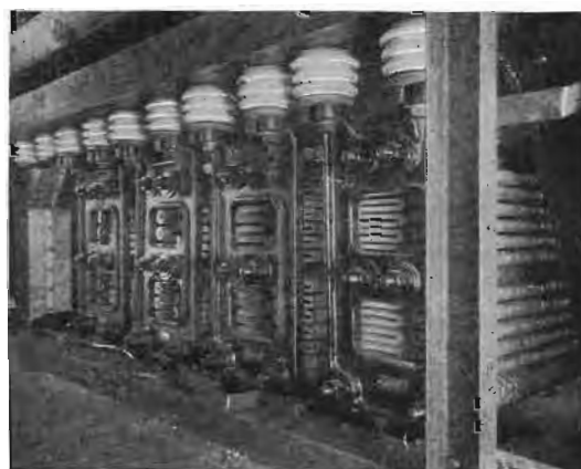
Fig. 17. View of 3000-volt Accelerating Grids Showing Method of Hanging
