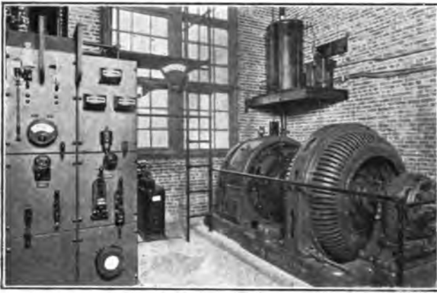
GREAT FALLS TERMINAL ELECTRIFICATION— SUBSTATION EQUIPMENT
