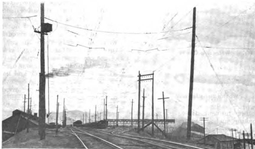
Fig. 9. View of the Contact System at the Stock Bin Yard
