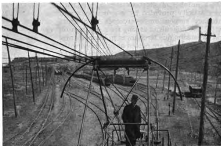
Fig. 8. Pantograph in Contact with Six Trolley Wires at a Switching Point
