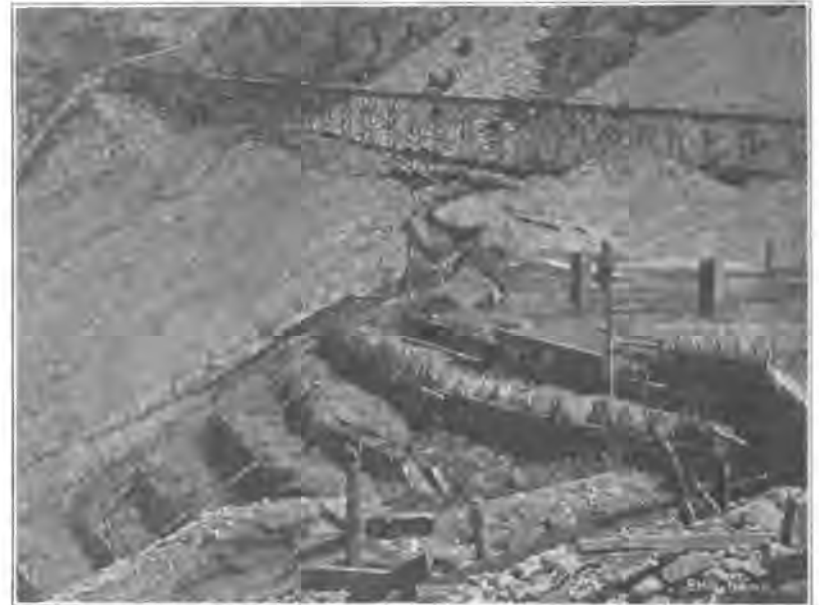
FIG. 9. BRUSH AND POLE DIKES FOR BUILDING UP THE SLOPE OF THE BANK.
