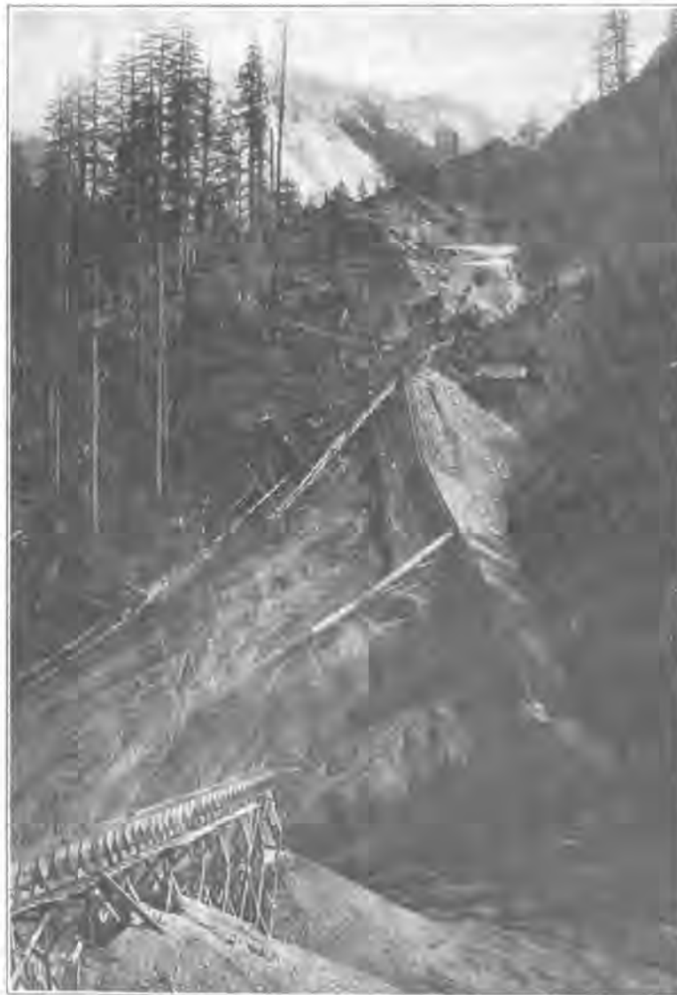
HYDRAULIC EXCAVATION AND SLUICING FOR CUT AND BANK AT TOPOGRAPHER'S GULCH; C., M. & P. S. RY.
