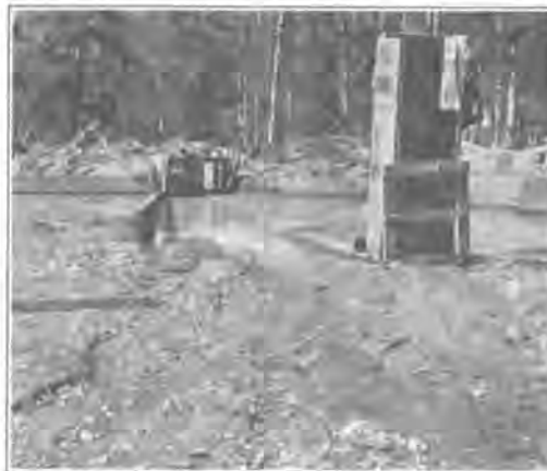
Fig. 10. Vertical Drain or "Chimney" for Draining Water from the Settling Pool Through the Bank.
