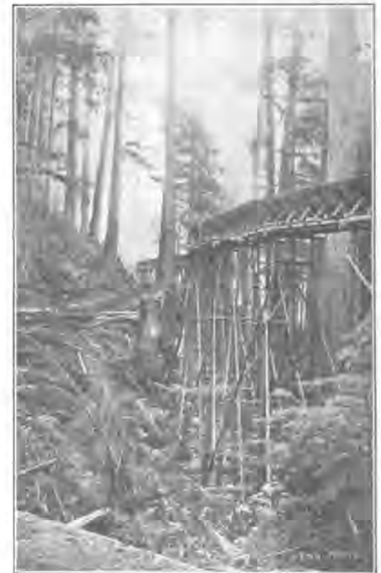
Fig. 3. V-Shaped Flume for Supplying Water-Power Pumping Plant for Hydraulic Excavation (Section 6 x 6 Ft.).
