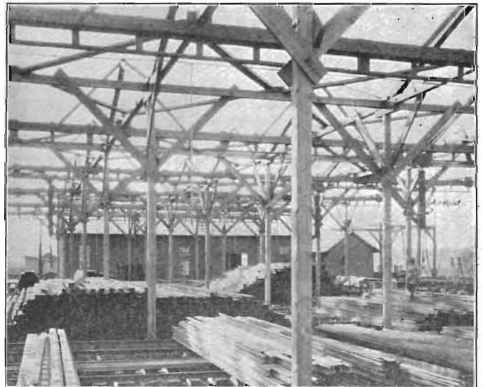
Chicago, Milwaukee & St. Paul Rail Yard, at Savanna, Ill.; Rail Mill in Background.
